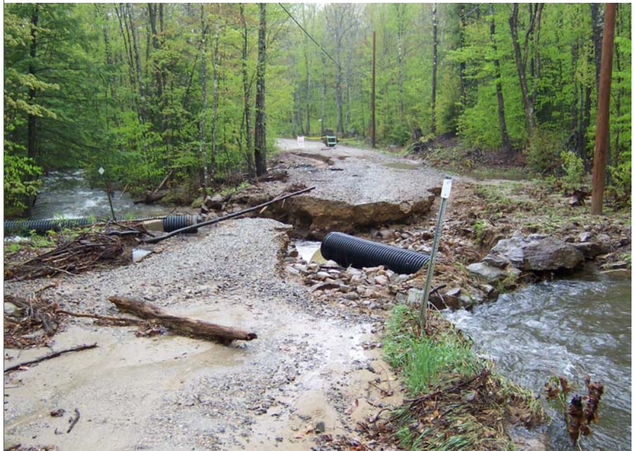
Infrastructure failure like this will be more common in the future due to more intense storms resulting from climate change. Attend our workshop on stormwater management and climate change to learn more.
